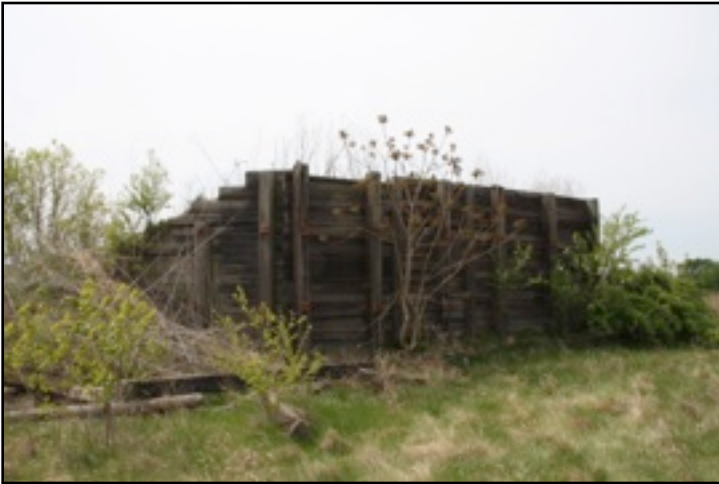
Fig. 7 - This photo and Fig. 8, from the present, show the deteriorated state of the ramp and this view gives a good view of the east wing. Note the placement of the visible anchor bolts is level with those in the front wall.
