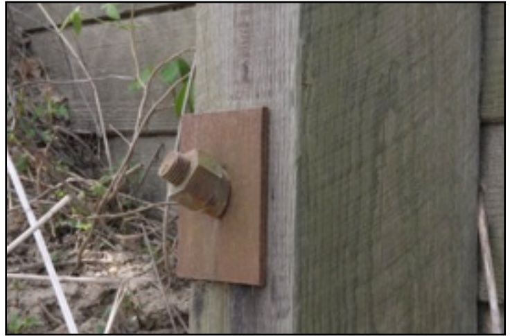
Fig. 4 - One of the anchor bolts with the plate and angled washer. There are two in each of the vertical front wall 10" x 10" timbers and in the vertical timbers of the wings.
