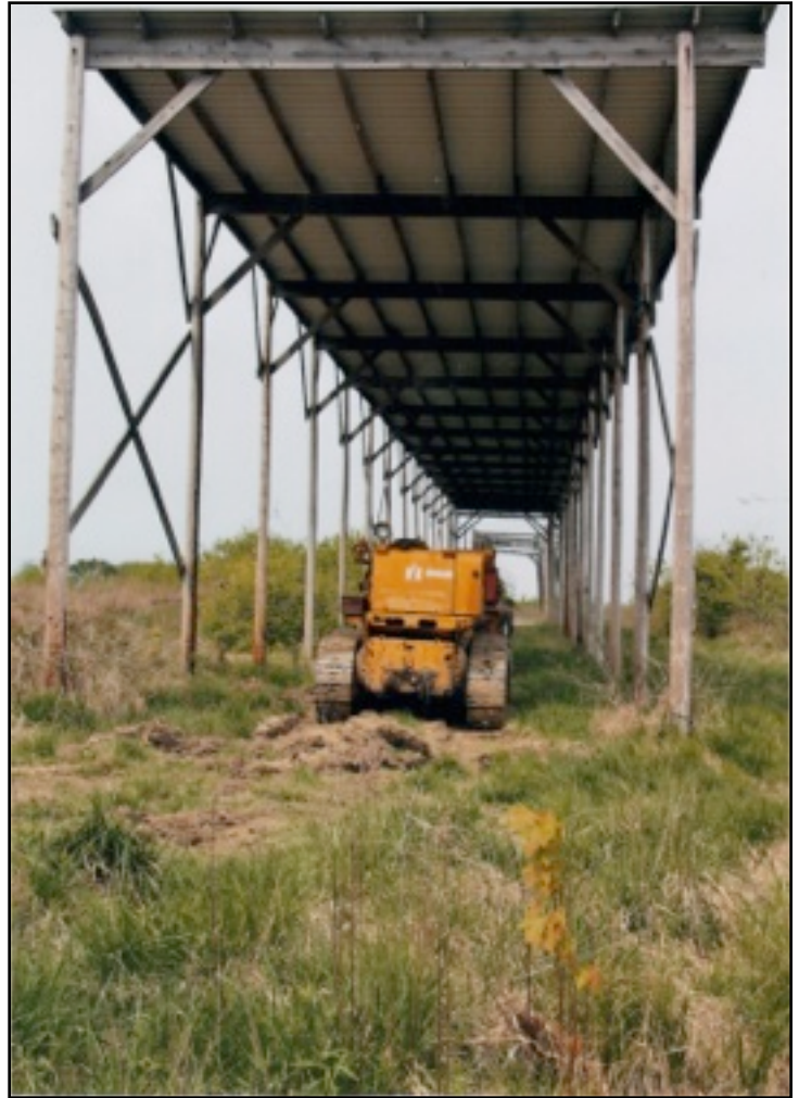
Fig. 14 - This is the end view of the new shelter with the deteriorated older shelter in the background. The view is to the west and to the right of the earth mover in the distance is the remains of the ramp for loading hoppers. This photo show the roof overhang on the right that is not present on the left. It also shows the spacing of the longitudinal roofing supports.
