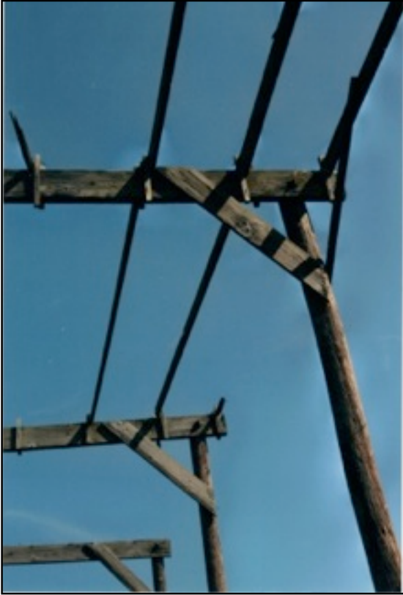
Fig. 13 - This contemporary photo shows the state of deterioration of the early section of the shelter. It also show well how the roof supports were attached.
