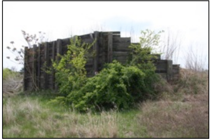
Fig. 8 - Here is the view with the west wing. More of the wing is visible. Note here also the placement of the visible anchor bolts is level with those in the front wall.
