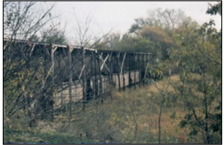
Fig. 11 - A 1988 view of the now deteriorated shelter from the loading ramp. Not noted on the drawings is what appears to be metal strips from the corrugated roofing down the sides of the poles. Perhaps for helping secure the roofing.
